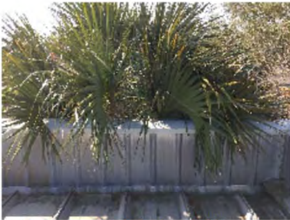
Tree overgrowth in the Southwest building corner
