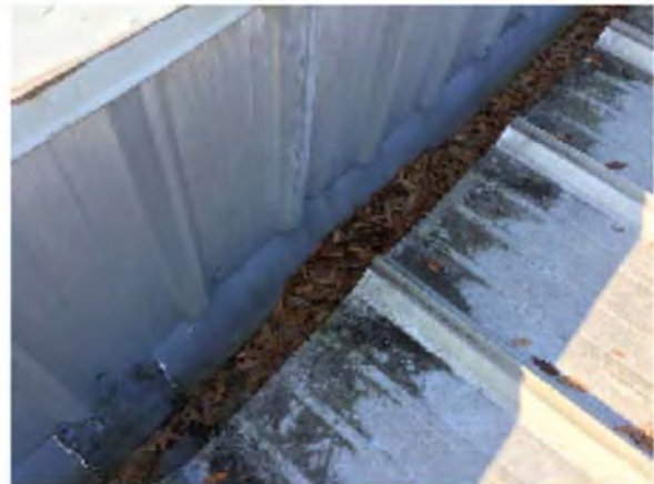
Leaves filling gutters and downspouts
