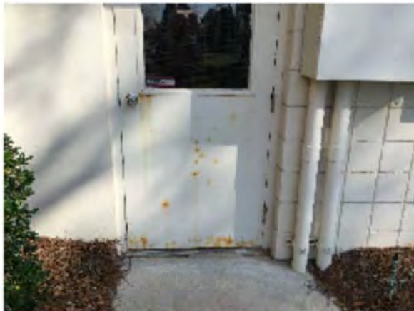
Oxidation of exterior steel doors on the South elevation
