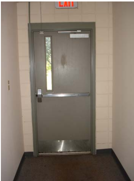
Existing Exit Door
