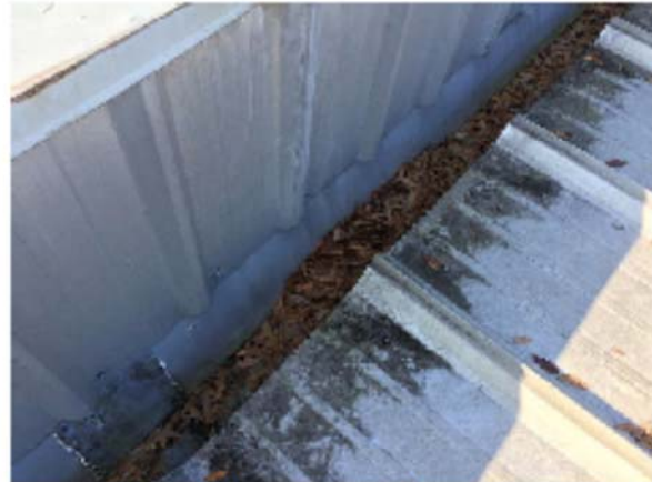
Leaves filling gutters and downspouts
