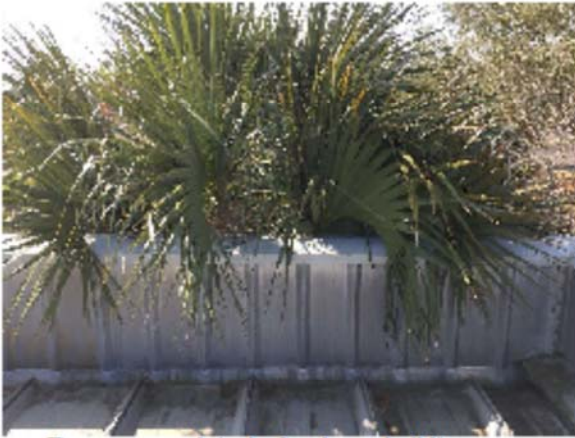
Tree overgrowth in the Southwest building corner
