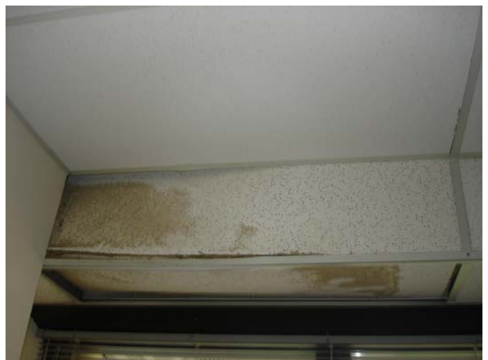
Existing Water Damage
