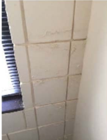
Moisture damage on interior of building
