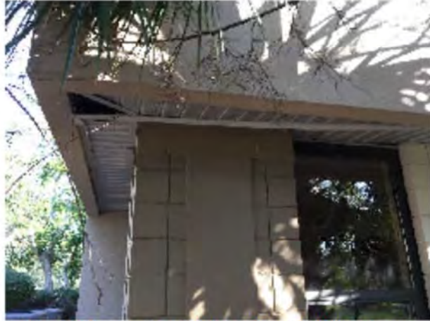
Typical damage to soffits in southwest building corner
