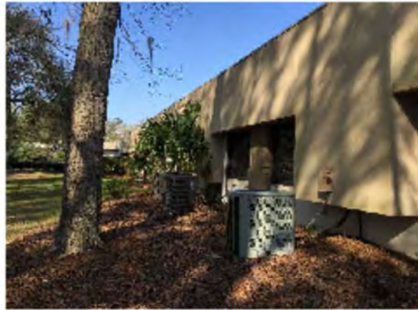
Trees growing into the exterior walls on southern elevation
