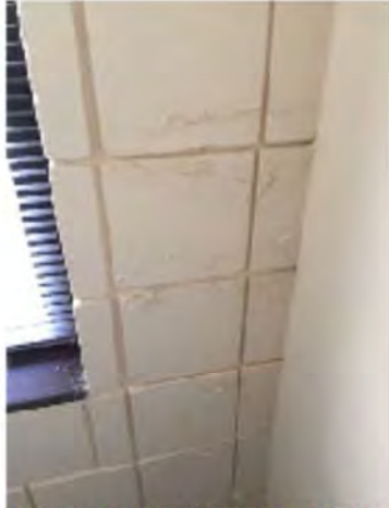
Moisture damage on interior of building
