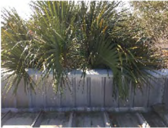
Tree overgrowth in the Southwest building corner
