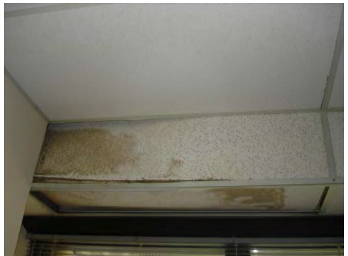
Existing Water Damage
